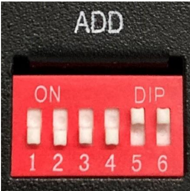
Figure 5-8: Example: Dip switch on BMS Rack 1
