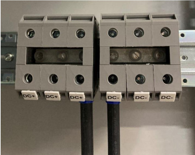
Figure 5-3: DC terminals on CombinerRack
